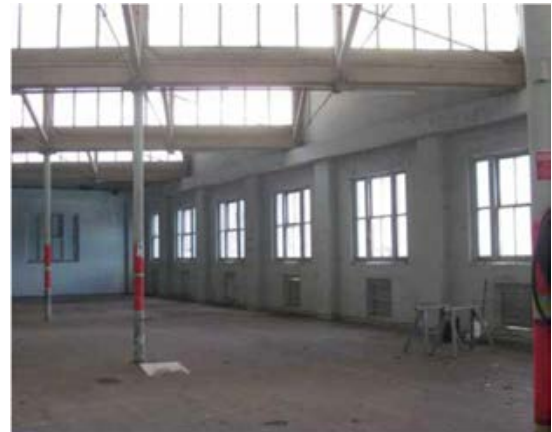
Top floor interior of 45 Jones Street (Ultimo Trade Centre) c. 2010 Source: OCP Architects P/L
